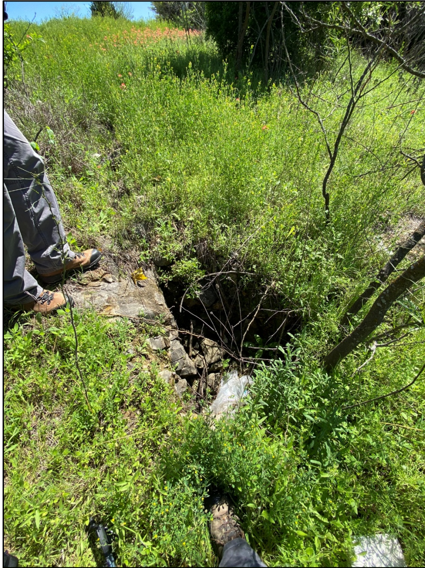
Feature Photo MPS-31 Non-karst Closed Depression. This closed depression is likely related to the existing utility line. No bedrock exposures are present within the depression.
