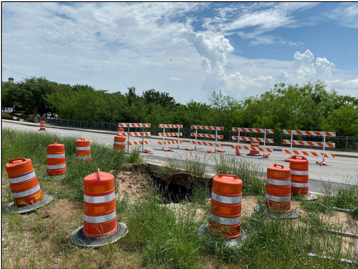
Feature Photo MPS-33 Non-karst Closed Depression (Photo 1 of 3). Traffic barriers were in place surrounding the hazard. Photo taken on April 8, 2020.
