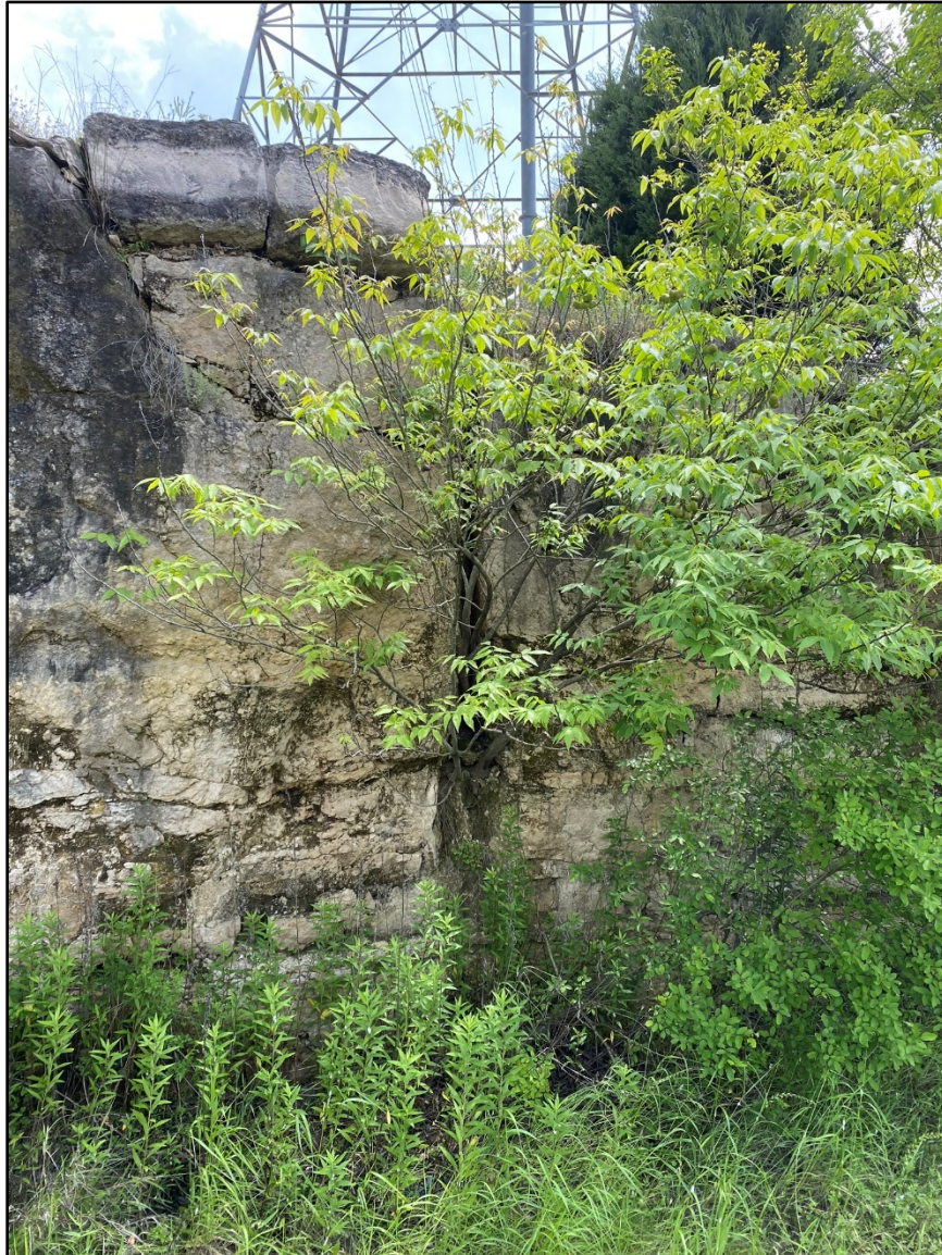
Feature Photo MPS-23 Solution Enlarged Fracture (Photo 1 of 2). Facing east at the cliff face. Southbound State Loop 360 is to the left.
