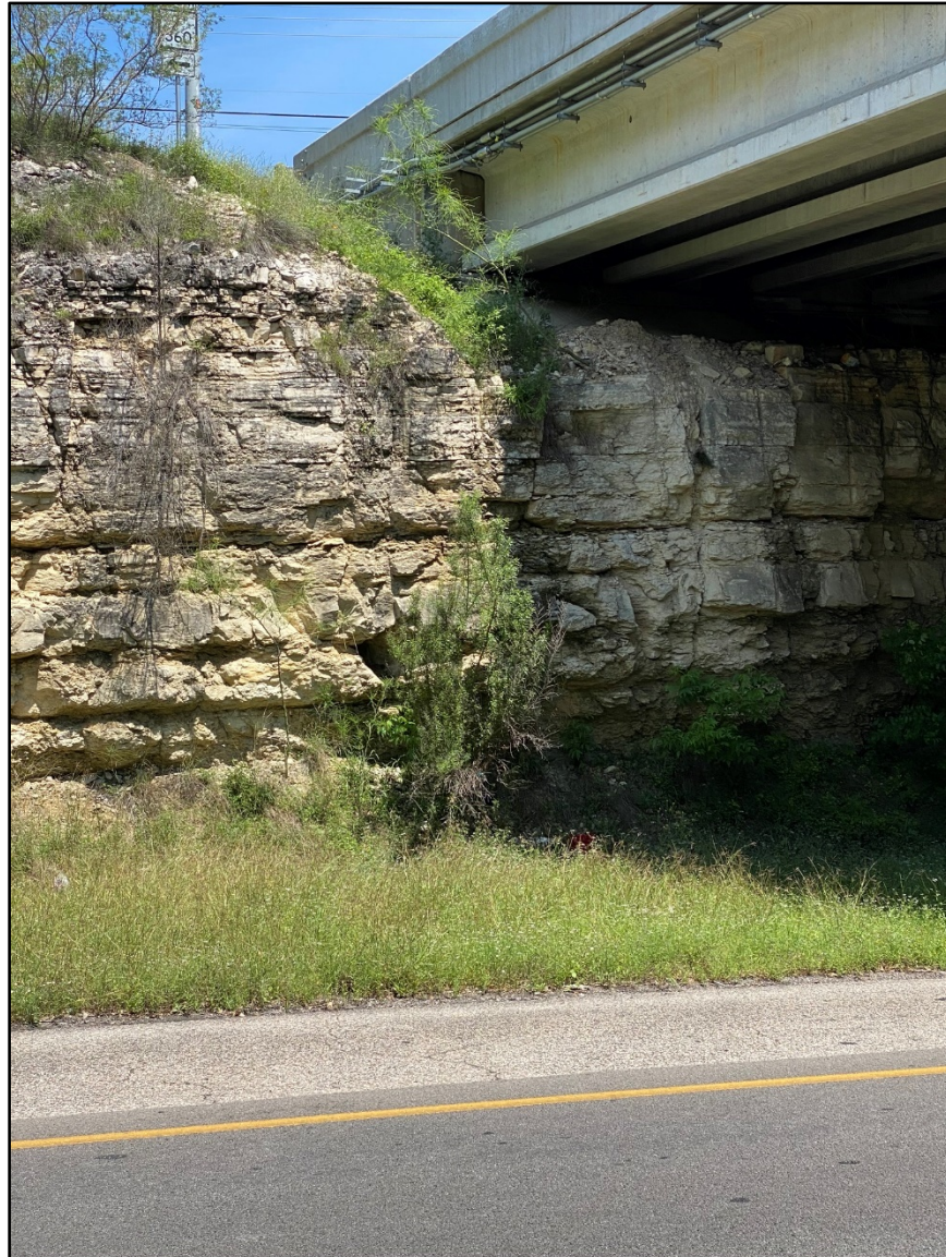
Feature Photo MPS-20 Solution Enlarged Fracture (Photo 1 of 2). This feature consists of a fracture with a solution cavity along a cliff face.
