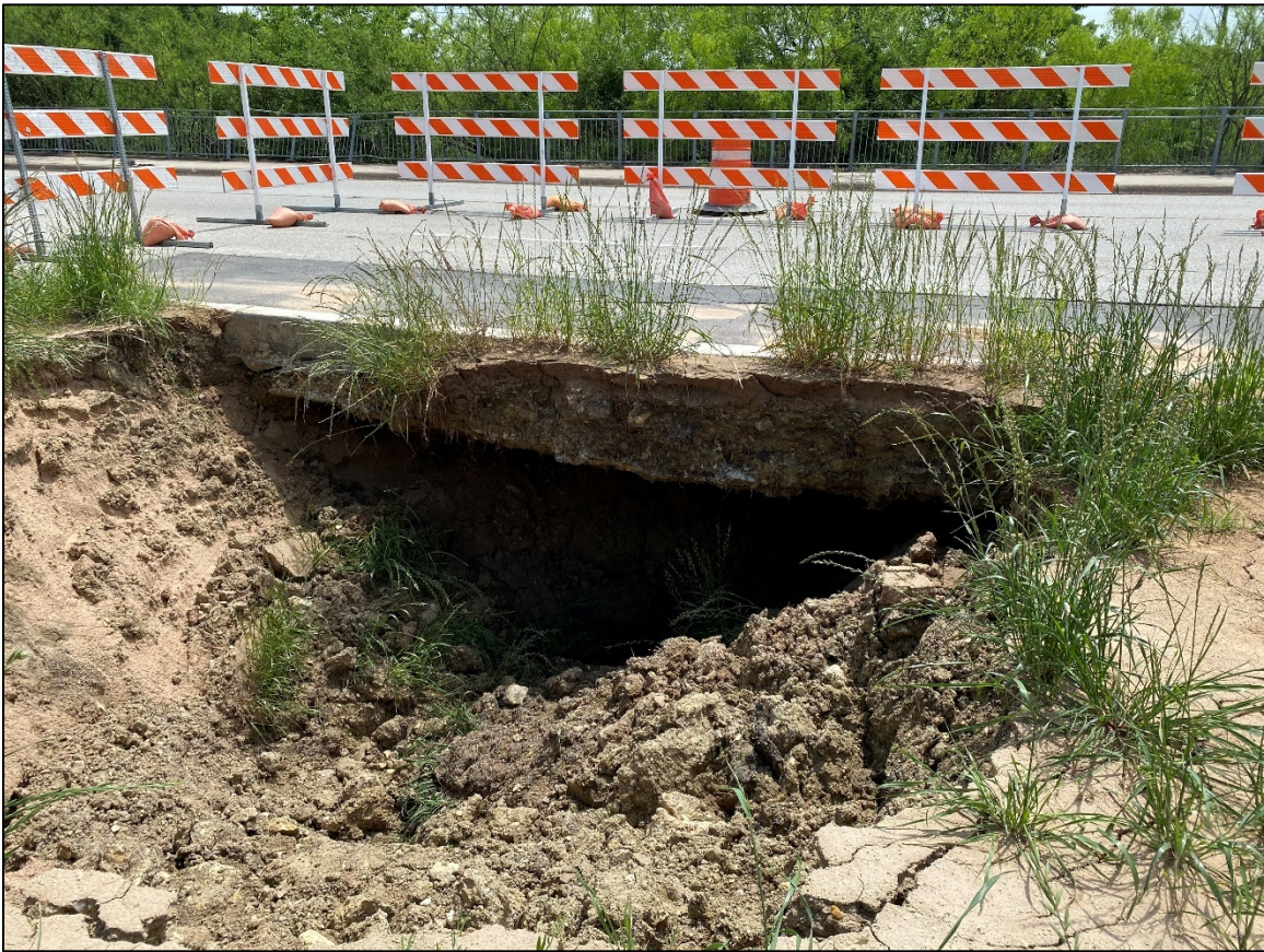
Feature Photo MPS-33 Non-karst Closed Depression (Photo 2 of 3). The depression was not excavated or probed due to the risk of further collapse. Photo taken on April 8, 2020.
