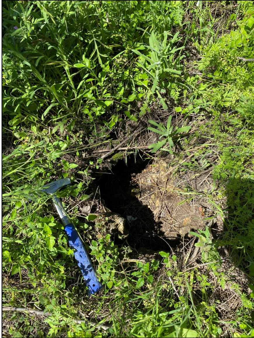
Feature Photo MPS-30 Non-karst Closed Depression. This closed depression is likely related to the existing utility line. No bedrock exposures are present.
