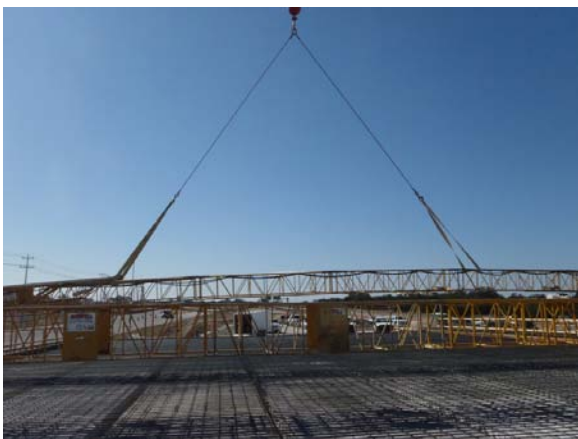
Preparations for placing concrete on a bridge deck at New Hope Drive
