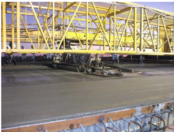
A smoothing and leveling device in action on the freshly placed concrete
