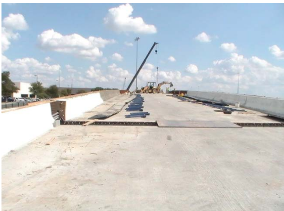
Roadway surface work on the West to North Direct Connector (Looking South)
