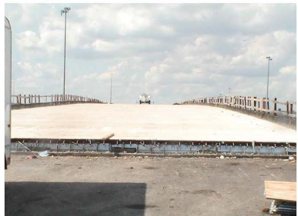
Roadway surface work on the East to South Direct Connector (Looking North)
