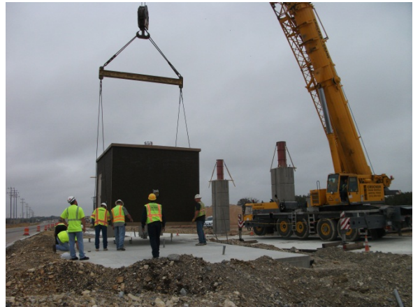
Precast concrete building for tolling equipment at the Crystal Falls on ramp
