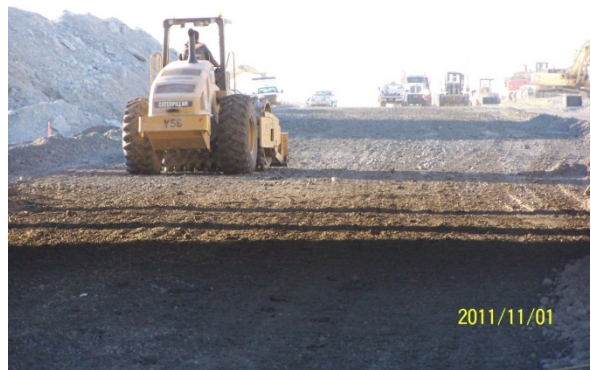
Compacting the final lift of soil on the 183A mainlanes south of Scottsdale Drive
