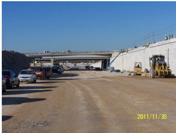
From the depressed 183A mainlanes, looking south at the Scottsdale Drive bridges
