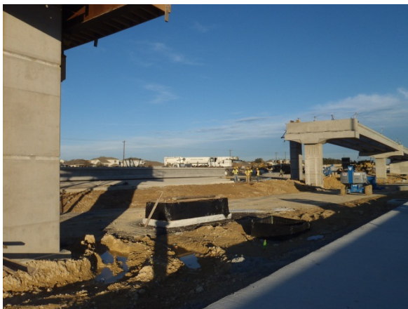
Future entrance ramp bridge and exit ramp overpass between New Hope and Scottsdale
