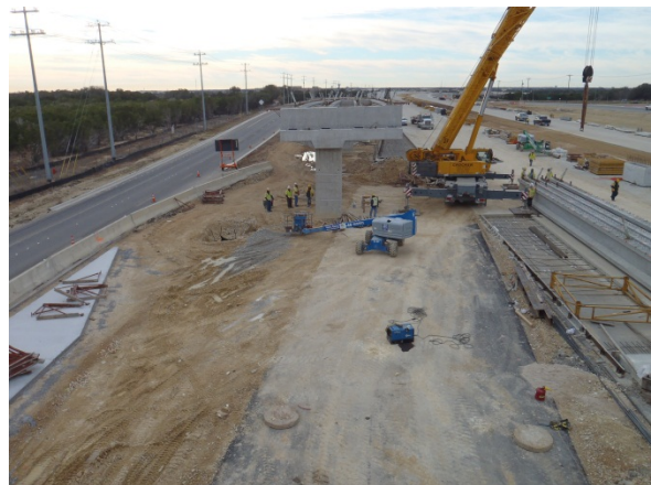
View from end of future bridge of braided ramp north of New Hope Drive
