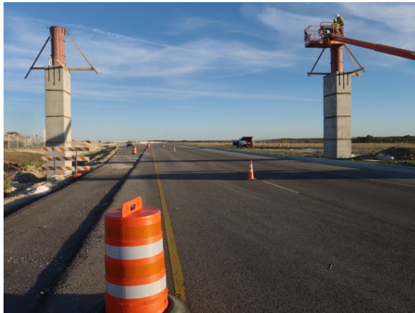
Overhead sign support columns spanning the frontage roads at the project's northern end
