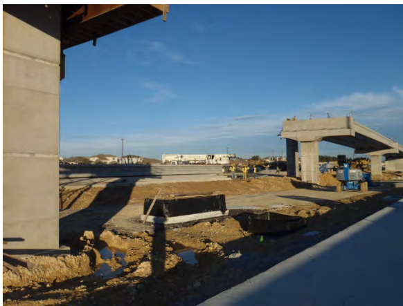
Future entrance ramp bridge and exit ramp overpass between New Hope and Scottsdale
