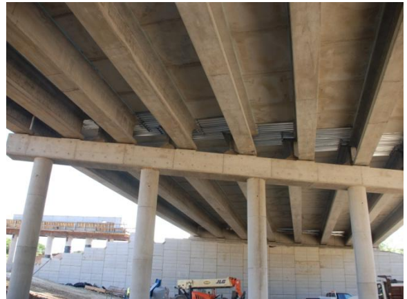
Eastbound frontage road bridge at Trib #5 and Wall S1-15 below (Looking East)
