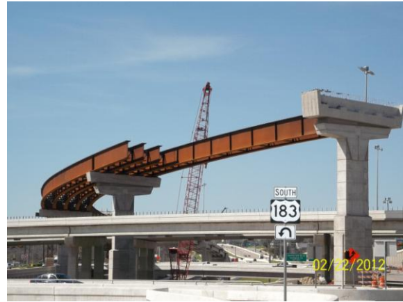
Steel Girder Erection on the South to East Direct Connector (Looking North)
