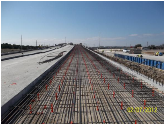
Approach Slab CRCP Construction along South to East Direct Connector (Looking West)
