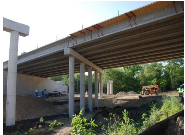
Bridge and retaining wall construction for eastbound frontage road at Trib #5 (Looking South)
