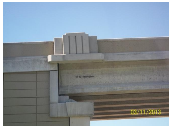
Bridge Identification Number installed on the North to West direct connector (Looking Southeast)
