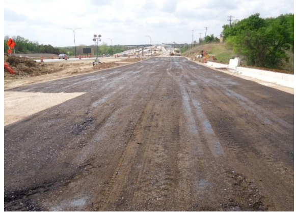
Placement of prime coat on the cement-treated base near MOKAN (Looking West)
