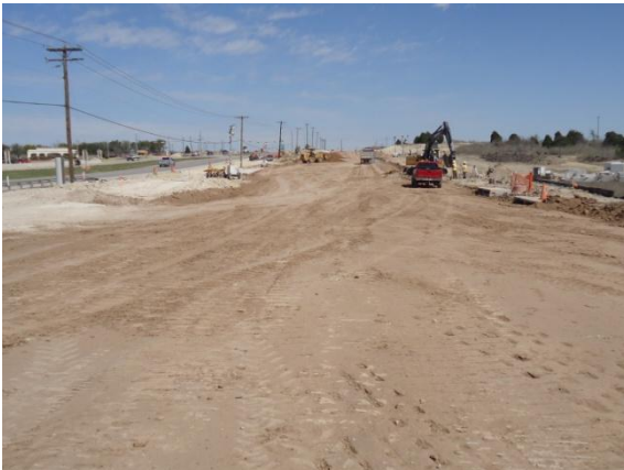
Embankment for the eastbound frontage road near Harris Branch Pkwy (Looking East)
