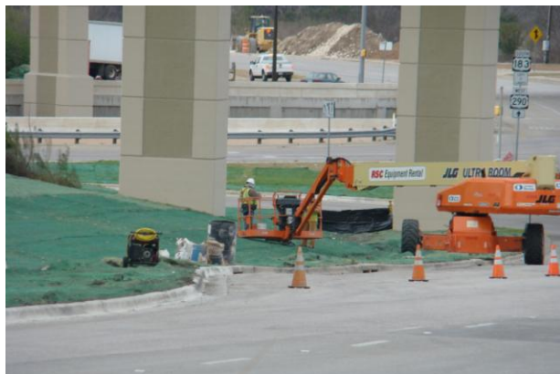
Repair of minor aesthetic blemishes on the West to South direct connector (Looking West)
