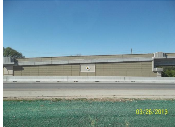
Completed MSE Wall with CTRMA Logo installed on the East to South Direct Connector (Looking Southwest)
