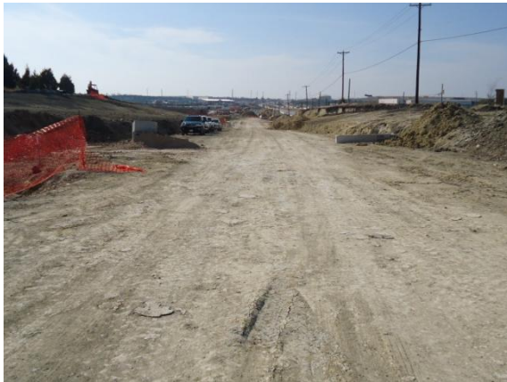
Excavation for the eastbound frontage road near Harris Branch Pkwy (Looking West)
