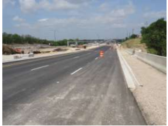
Construction of the eastbound frontage road east of Chimney Hill Blvd (Looking West)
