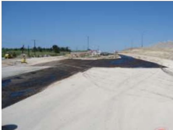
ATMOS metering station at eastbound frontage road near Parmer Lane (Looking East)
