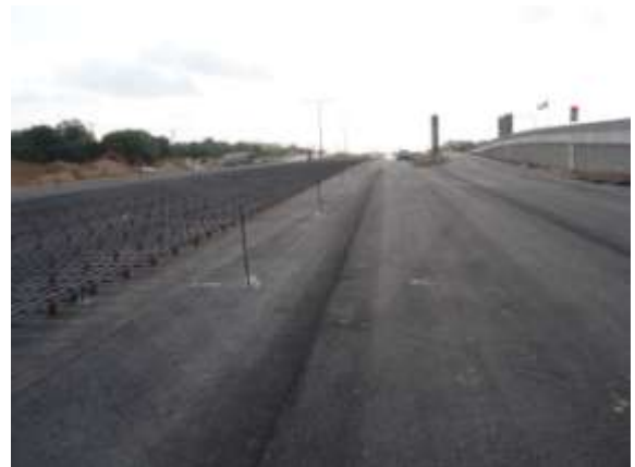
Tied steel for concrete pavement between Arterial "A" and Giles Road (Looking East)
