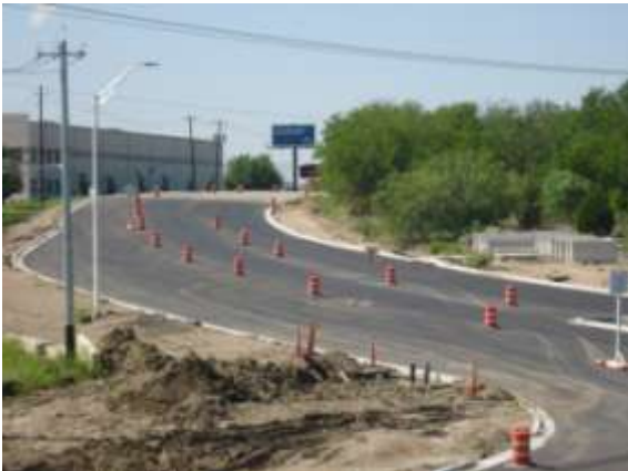
HMA has been placed at the Johnny Morris Road intersection (Looking South)
