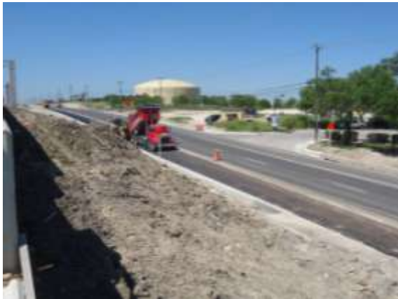
Asphalt Base on the westbound frontage road west of Giles Road (Looking Northwest)
