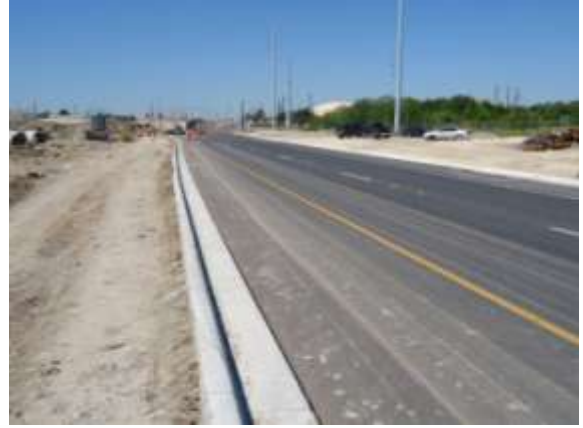
Asphalt Base on the westbound frontage road east of Giles Road (Looking West)
