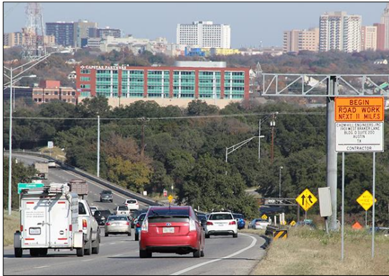
Road construction signs were installed in December on the MoPac Improvement Project
