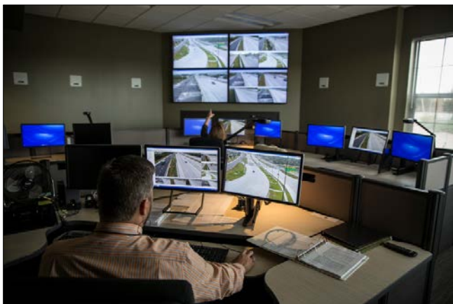
Mobility Authority Traffic Management Center
