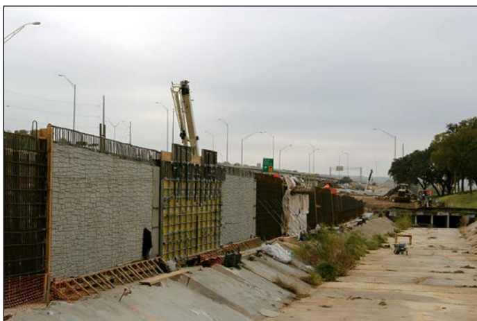
Retaining Wall Construction near Lake Austin Blvd Exit and Johnson Creek Trail – Nov. 20, 2014
