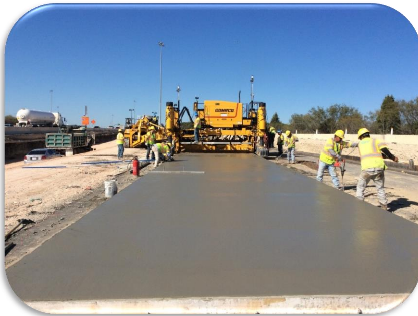
Roadway Paving Northbound Main Lanes Beginning of Project to Manor/Springdale Road [December 1, 2016]
