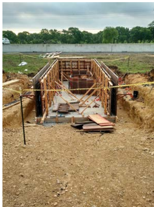
At GS1: Splitter Structure at Pond A
