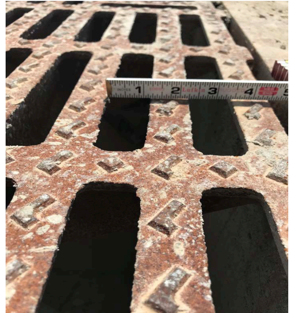
Drainage Grate not ADA Compliant
