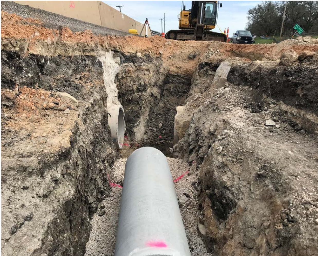
No Trench Protection
