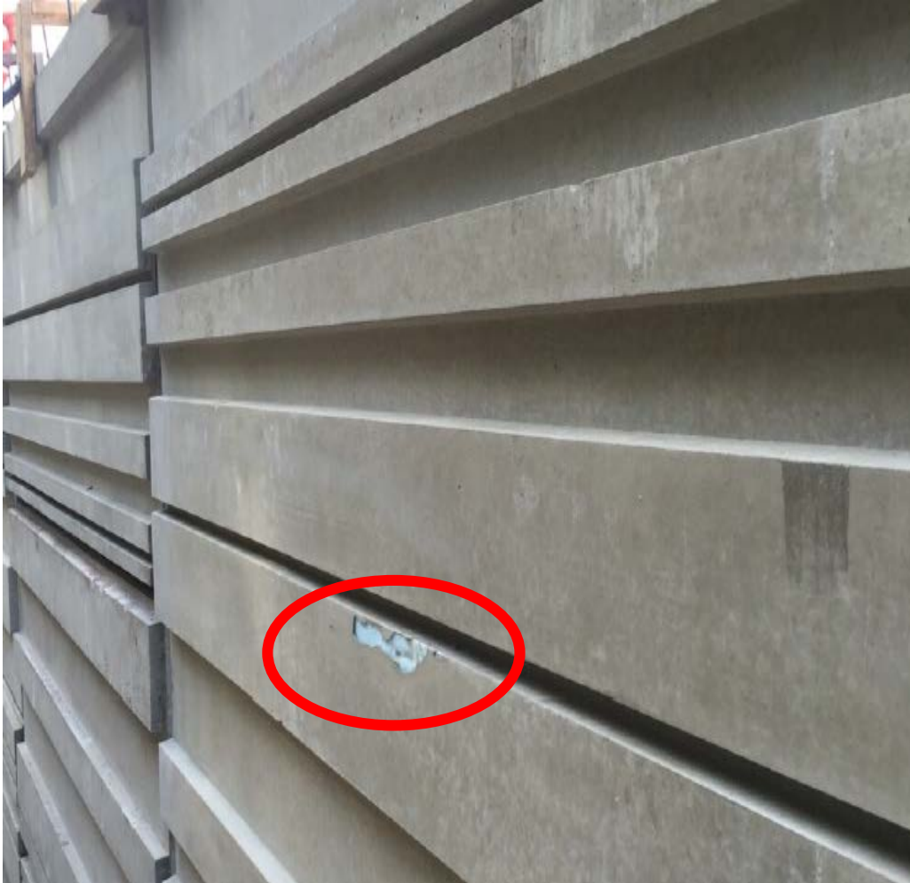
Exposed foam in wall panel
