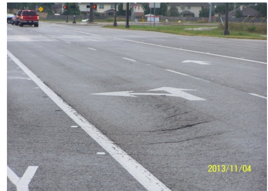
Observed fatigue cracking
