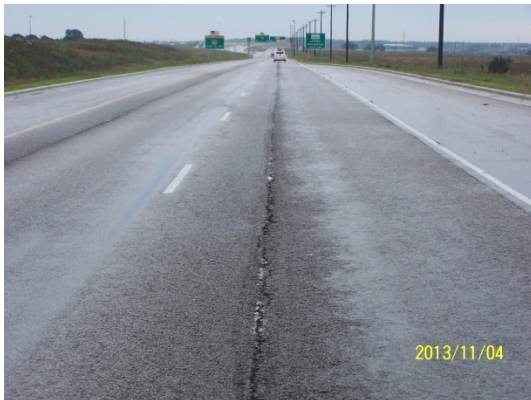
Observed longitudinal cracking
