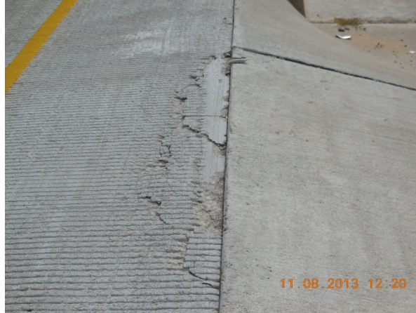
Concrete pavement spalling at northbound entrance ramp just north of New Hope Drive
