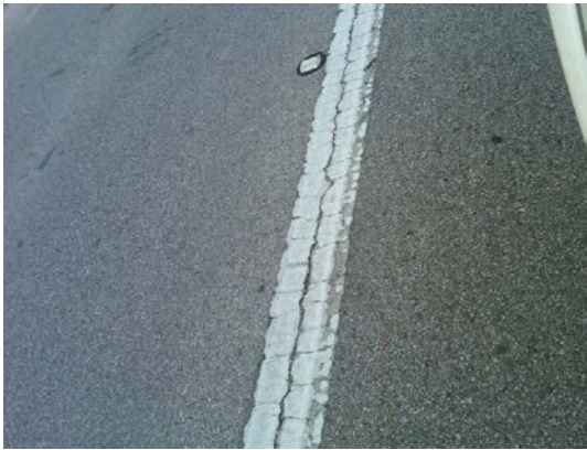
Observed pavement marking cracking
