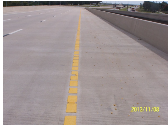
Observed pavement marking fading
