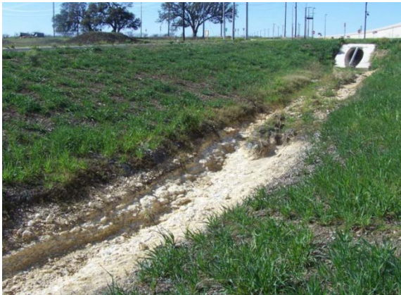
Observed channel erosion
