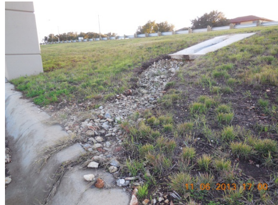
Erosion above retaining wall 20
