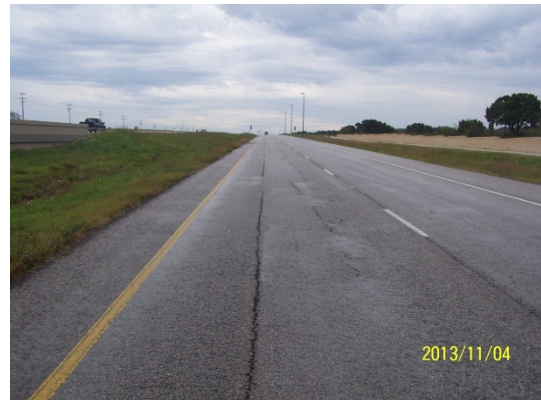
Observed longitudinal cracking
