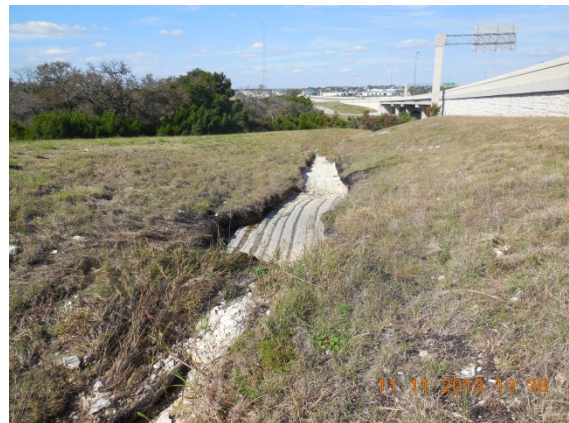
Erosion in channel along southbound mainline south of South Brushy Creek
