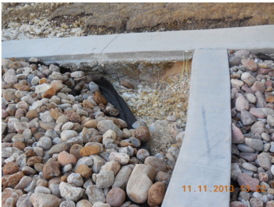
Erosion of decorative rock at the north end of the South Brushy Creek Pedestrian Bridge
