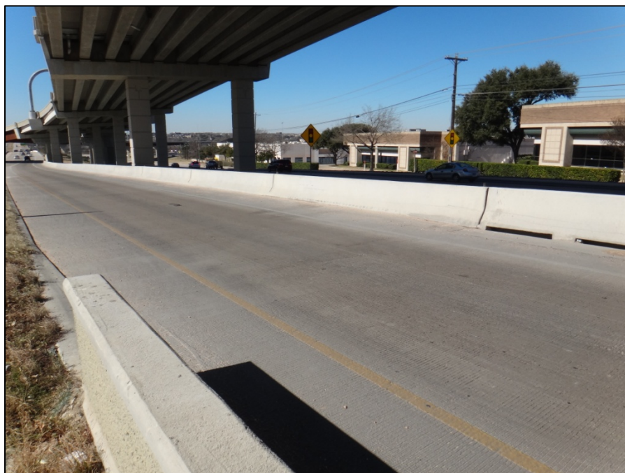
Faded white striping along westbound entrance ramp
