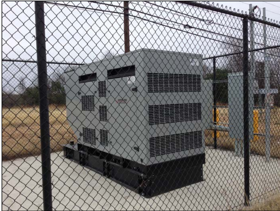
Emergency generator that serves both Ramps 1 and 2 toll locations
