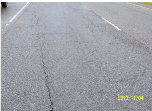
Observed fatigue cracking
