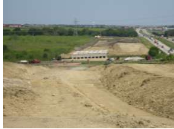
Excavation and Embankment for the westbound frontage road at Parmer Lane (Looking West)
