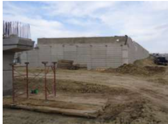
Erection of Wall S2-13 for the eastbound mainlane east of MOKAN (Looking East)
