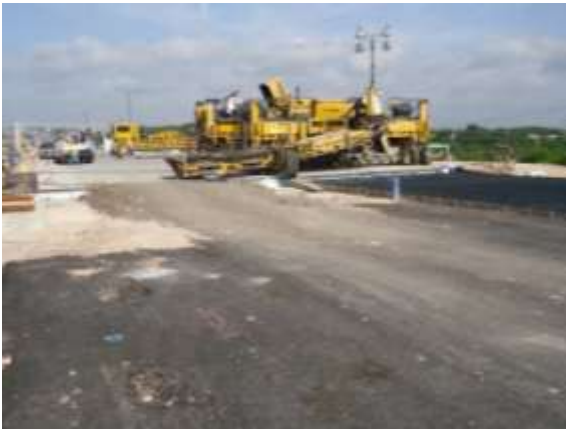
Crews continue to install concrete pavement on the eastbound mainlanes (Looking West)
