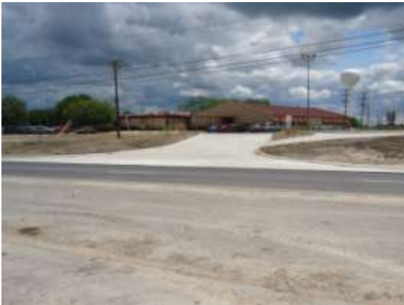
Construction of a new driveway at Manor New Tech High School (Looking South)
