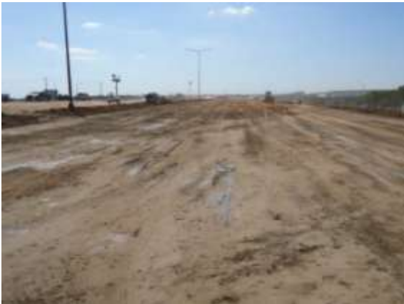
Construction of embankment for the westbound mainlanes near Harris Branch (Looking West)
