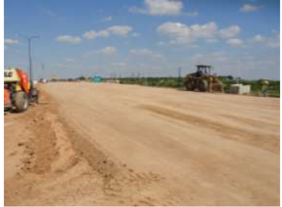
Construction of embankment for the eastbound mainlanes near Harris Branch (Looking East)
