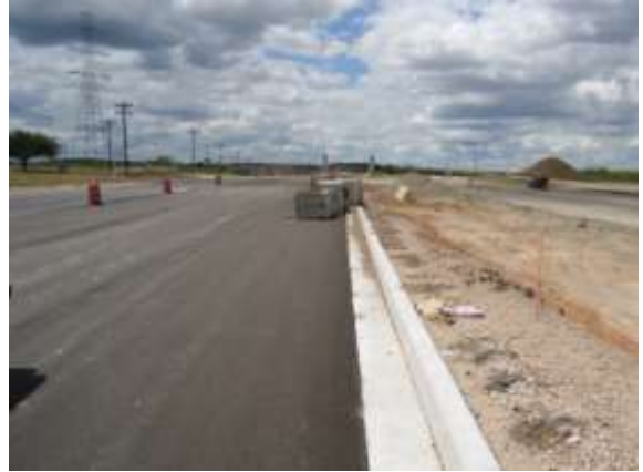
Curb and gutter has been poured west of Gilleland Creek (Looking West)
