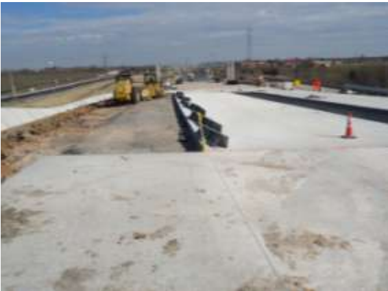
Crews continue to pour concrete paving east of Tributary #1C (Looking East)
