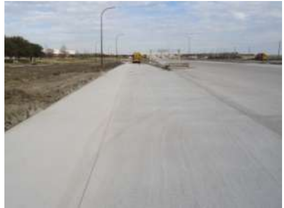
The westbound entrance ramp west of the SH 130 interchange is paved (Looking East)
