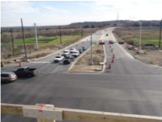
The final asphalt surface course has been placed at the Parmer Lane intersection (Looking South)
