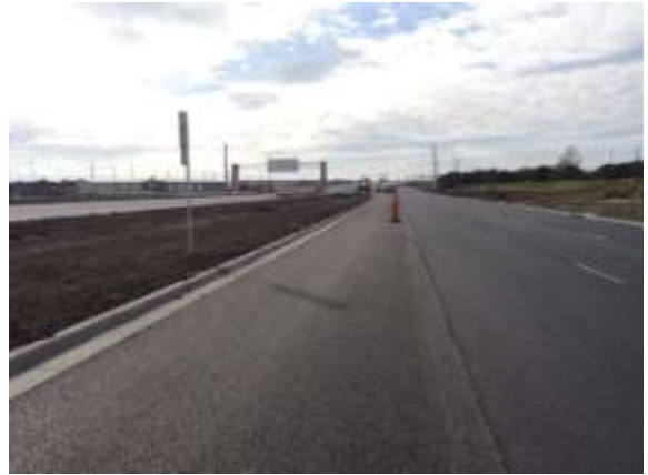
The final asphalt course has been placed east of Giles Road (Looking West)
