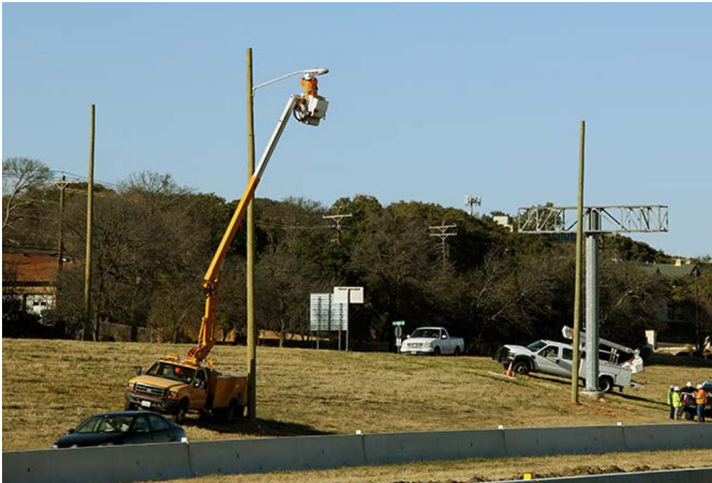
Temporary safety lighting system installation. The temporary lighting system will remain in place until the proposed lighting system is constructed.
