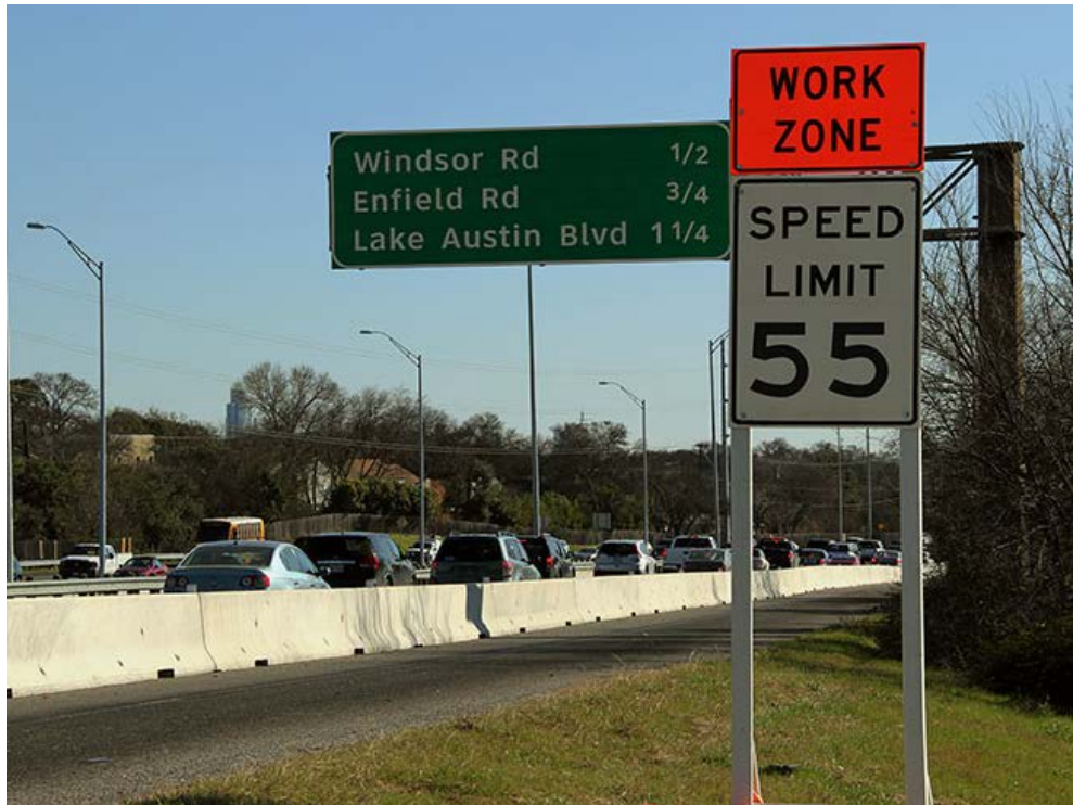
The speed limit has been reduced to 55 MPH along portions of the Project corridor.
