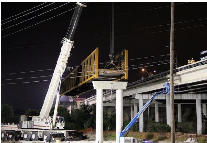
First span of 525-foot bike/ pedestrian bridge now in place over Union Pacific tracks southbound (April 9)
