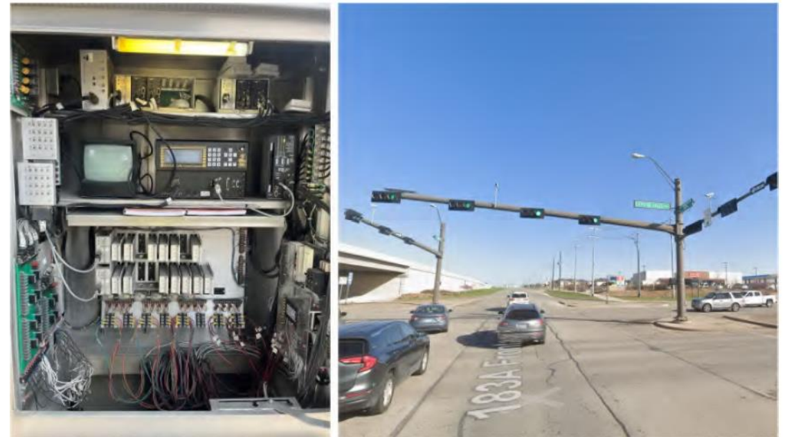
Figure 1: Existing signalization hardware and in-cabinet equipment for the 183A Toll and Crystal Falls Pkwy intersection.
