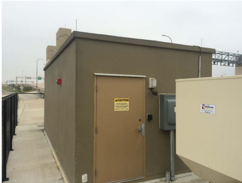
ILP building located at the Parmer Mainlane tolling location
