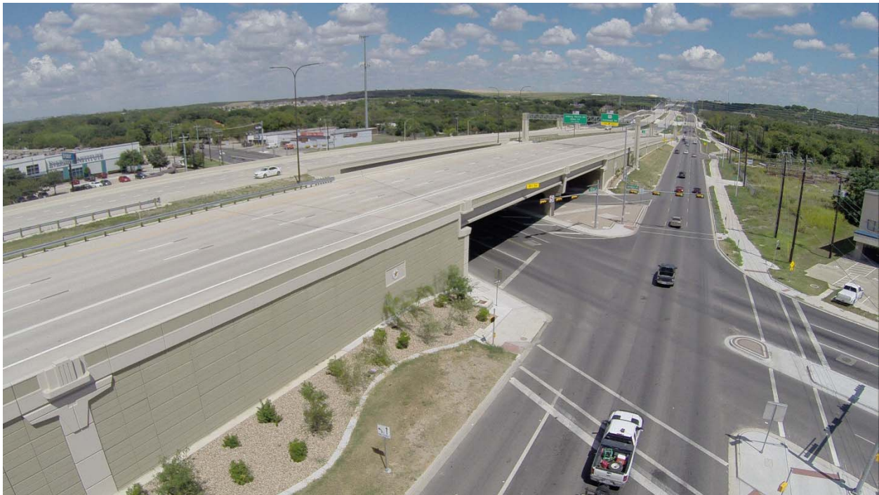
Retaining Wall S1-05 at the Southwest Corner of the Springdale Rd Intersection
