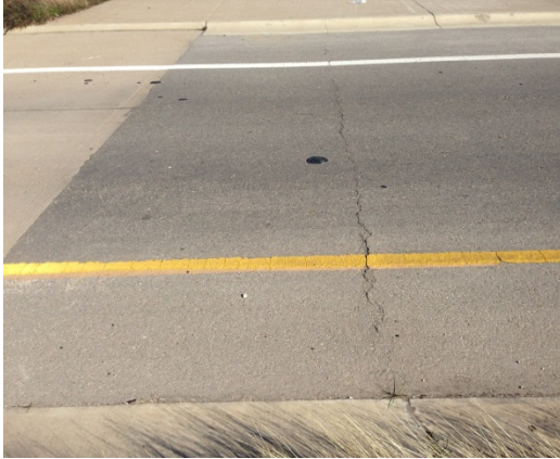
Observed Transverse Crack at Ramps
