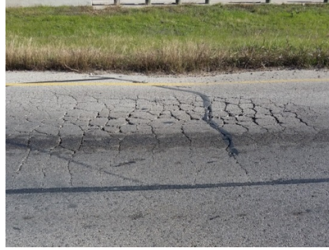
Southbound Brushy Creek Loop Alligator Cracking
