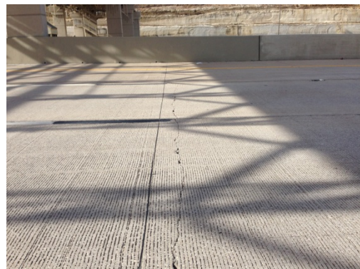
Observed Transverse Cracking
