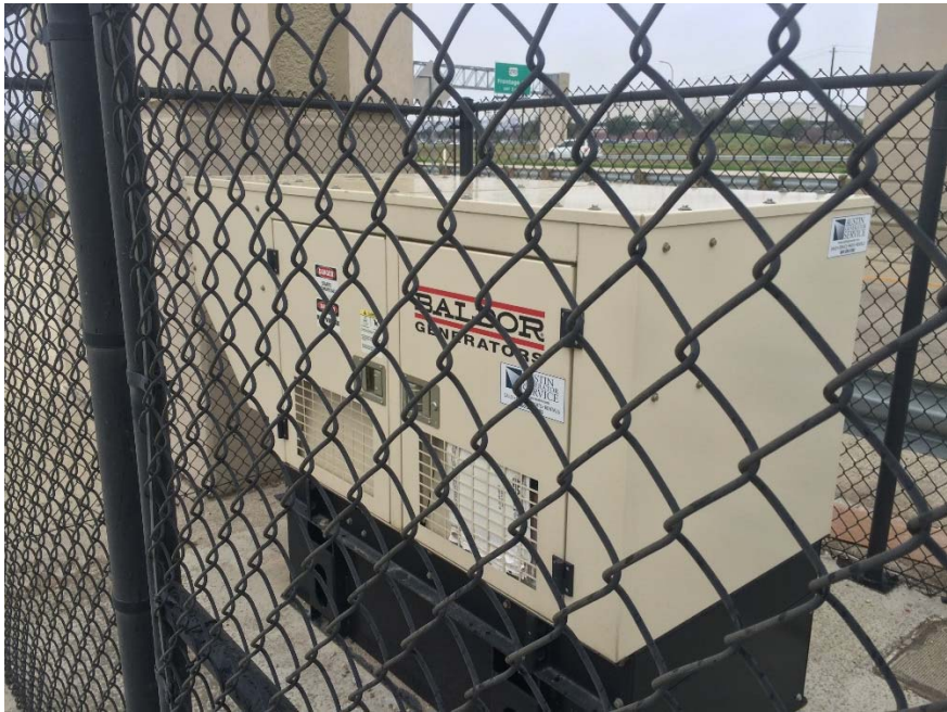
Emergency generator that serves the Eastbound Entrance Ramp toll location East of Johnny Morris Rd
