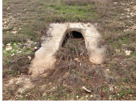
Clogged Inlet Pipe
