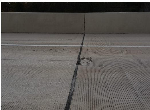
Observed Pothole on Brushy Creek ramp
