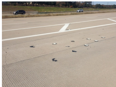
Observed Missing Buttons
