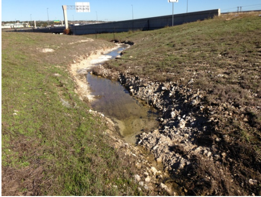
Erosion between SBML and SBFR
