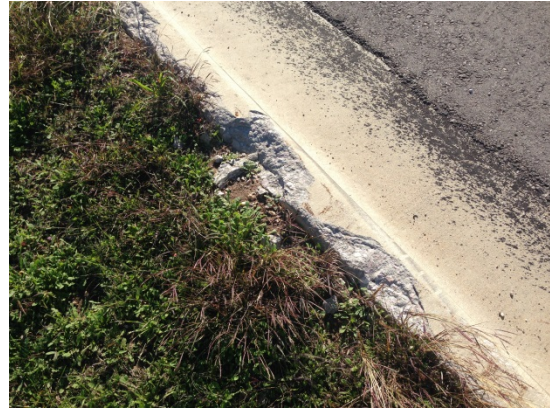
Observed Chipped Curb
