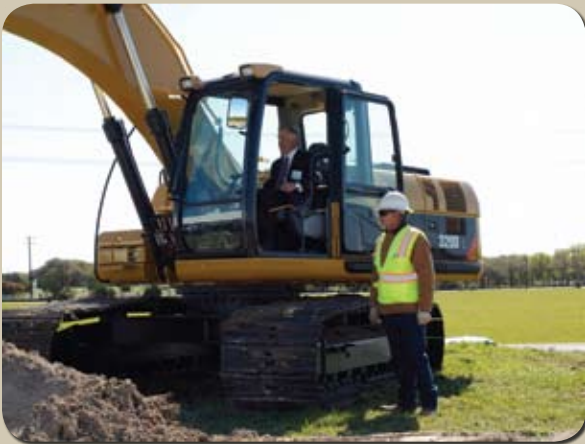
Mobility Authority Chairman Ray Wilkerson breaks ground on the 183A Northern Extension
